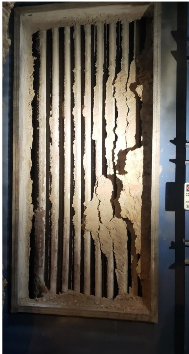
Before: normal fouling - heavy fouling @ 3 months - Vortex installed: 4 hours - all deposits left as-found
